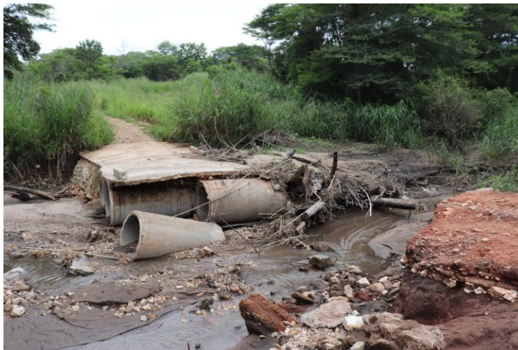
Figure 1: Image of a bridge washed away in Chipekete, Rufunsa District. Credit: Bernard Mwaba - JCTR
